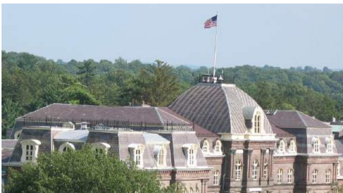
Figure 3: Dutch Lap slate roofing on the dome of the center wing of Main Hall, Vassar College, Poughkeepsie, New York, built c.1864.
