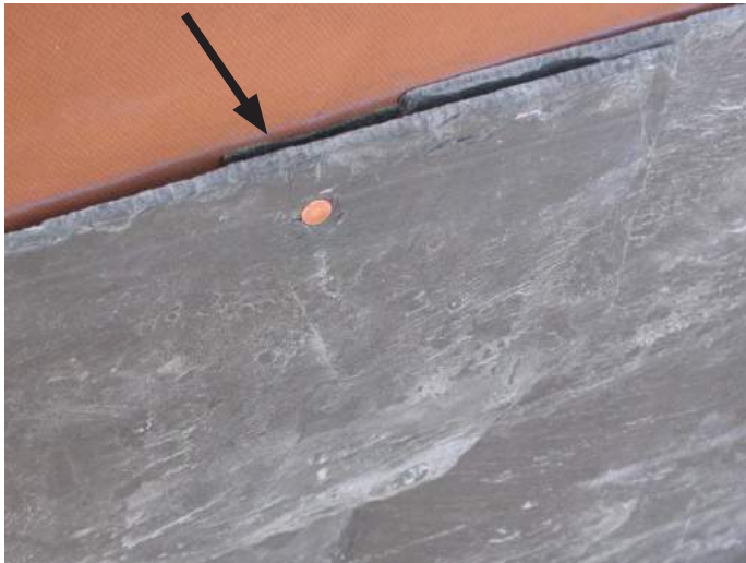
Figure 6: Just prior to the installation of each slate shingle, a 4” x 4” piece of self-adhering tape (see arrow) can be placed on the underlayment at each slating nail location to help seal around the nail holes.
