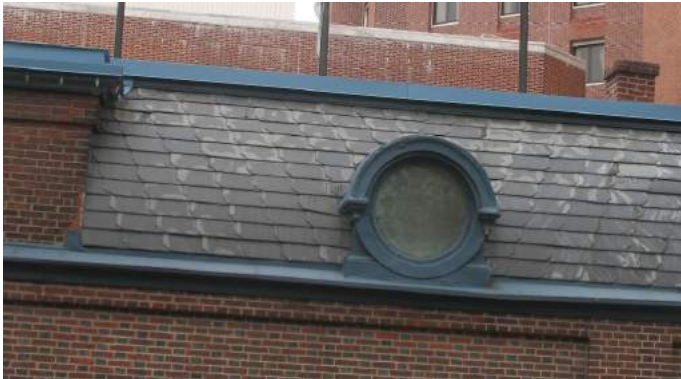
Figure 2: Dutch Lap slate roofing on the Pine Building entrance of the Pennsylvania Hospital, Philadelphia, Pennsylvania.
