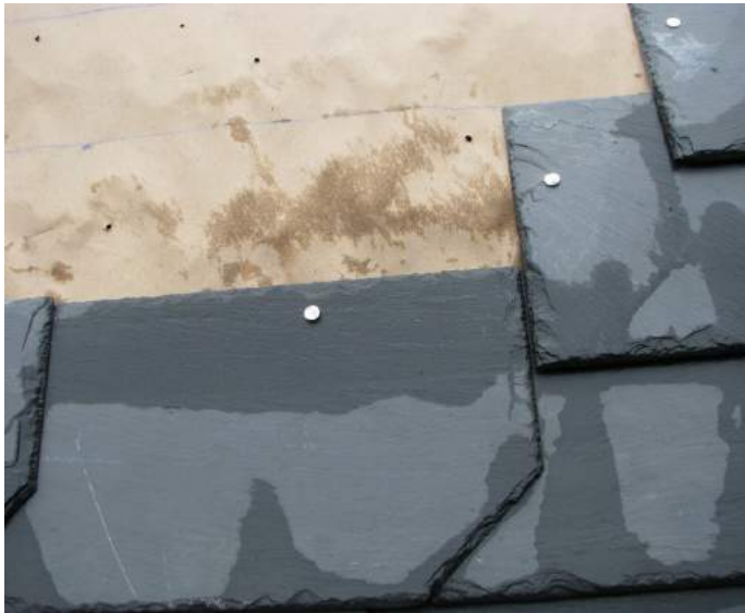
Figure 5: Water testing was carried out using a garden hose. Water was systematically sprayed at various angles (downward, straight on, at a slight side angle [i.e., into the side laps], and at an upward angle) for durations of three to five minutes. After each interval, slates were removed. When water was sprayed at a downward angle, the rosin paper was found to be dry. Some water did extend into the side and top laps of the slate, but not enough to reach the nail holes. When water was sprayed straight on and at side and upward angles (simulating wind-blown rains), areas of wetness on the underlying rosin paper were observed, and a significant portion of the concealed areas of the slates were wet, including areas around many of the nail heads (see image above)
