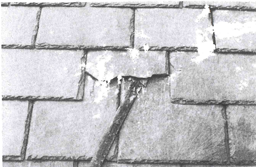
To remove the damaged slate, first hook the ripper on one of the two nails holding the slate.
