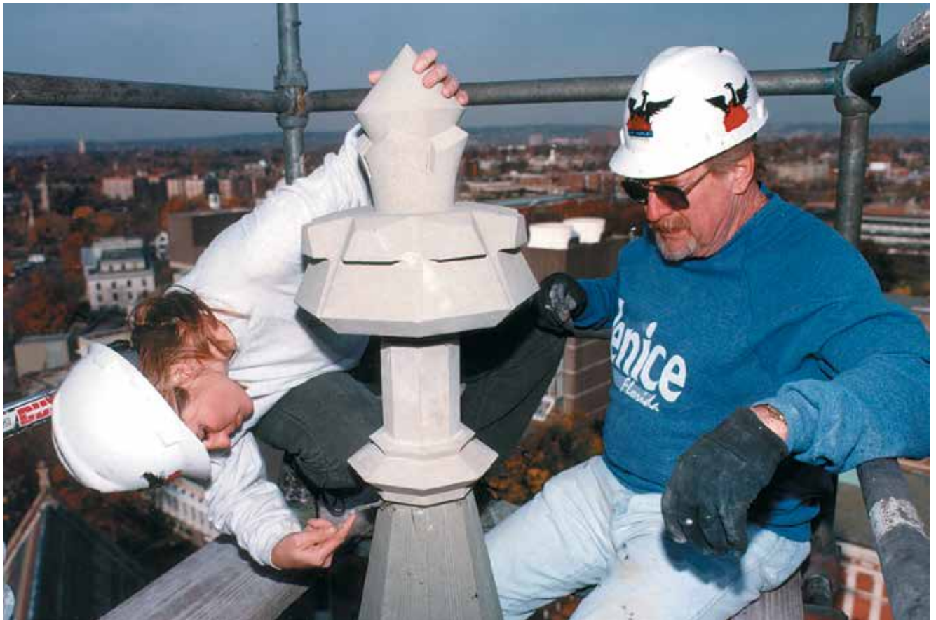
Approximately 50 or 60 stones were replaced during the restoration of the sandstone pinnacles.
