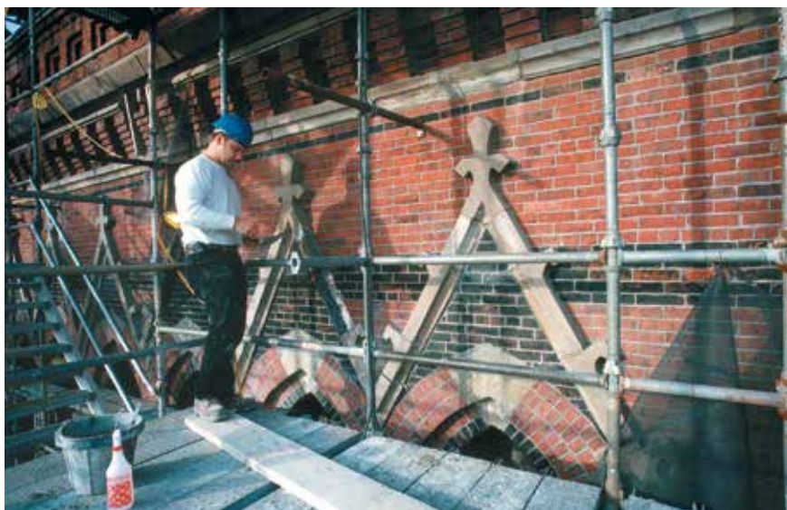
According to Dr. Judith E. Selwyn of Preservation Technology Associates in Boston, MA, the sandstone pieces with minor damage were tooled back to a new surface.
