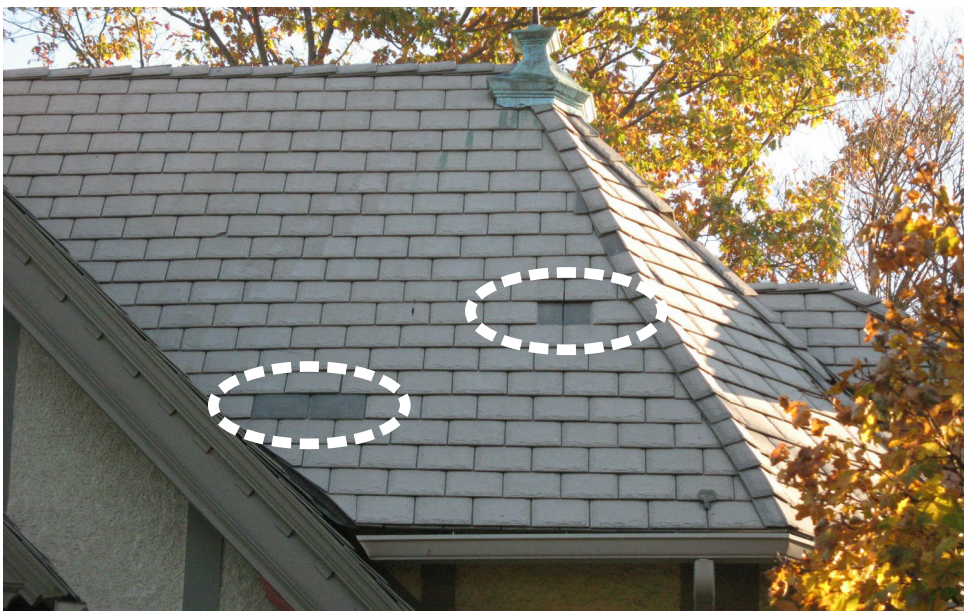
Figure 5: An example of fading color in synthetic shingles. In the center, a missing shingle exposes the normally concealed portion of two shingles in the course below. In the lower left, two new shingles highlight the fading that has taken place in the adjacent shingles over time.
