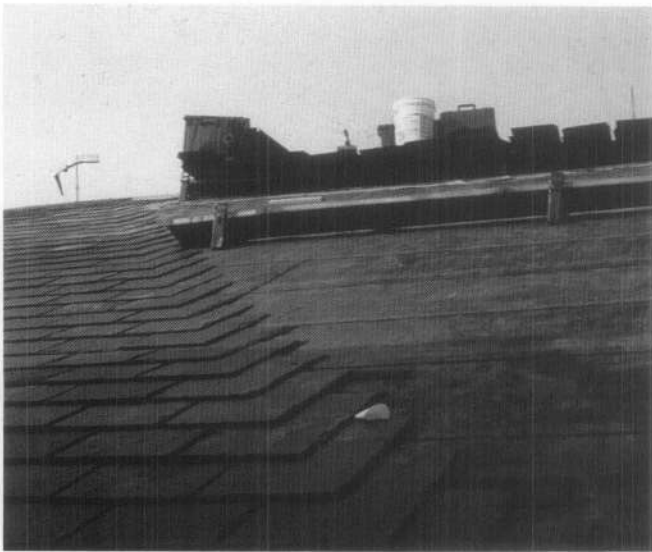
(h) This installation pattern allows the slates to be laid in courses leaving a temporary path of travel to avoid stepping on installed slates.
