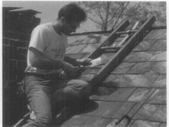
(d) A copper bib is formed to protect the newly created nail hole.
