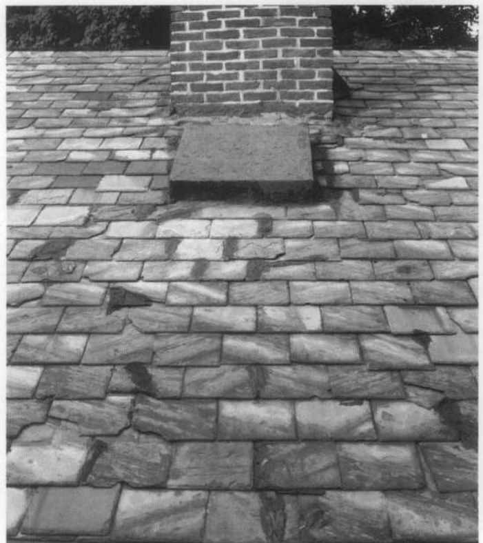
Figure 20. This roof has been poorly repaired numerous times in the past. The installation of mastic to seal out moisture has only exacerbated the problem. A timely repair and good maintenance could have extended the life of this roof.
