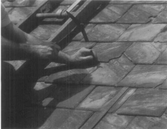
(c) A new slate is secured in place with a copper nail.
