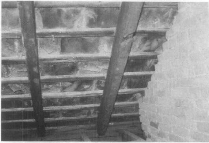
Figure 15. View of the underside of slates laid on open sheathing shows that delamination and flaking is just as bad or worse on the underside of slates as on the exposed surface. This is why most slates cannot be flipped over for reuse.
