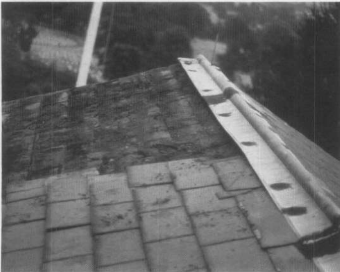
(c) Slate was removed in sections to avoid stress on timber framing.
