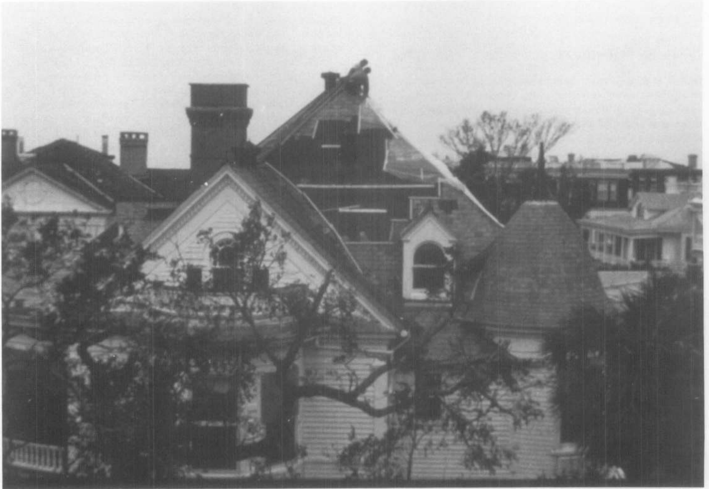
Figure 21. As a result of hurricanes and other disasters, it may be necessary to temporarily stabilize a roof until materials can be obtained and a qualified roofing contractor hired. Heavy roofing felt was stitched into this slate roof to stop moisture penetration until matching slate was obtained for repair. Significant slate roofs should not be stripped off and replaced with asphalt shingles. Photograph courtesy of the National Park Service.
