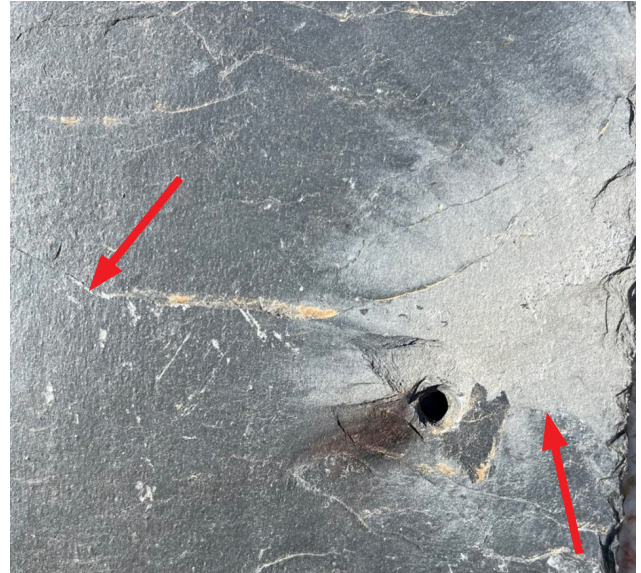
Figure 3: Discoloration (lightening; right arrow) and micro-cracking (left arrow) occurred in this slate shingle due to the heat generated when lightning struck one of its copper nails. 9 (Photo courtesy of John Chan, The Durable Slate Company, Savage, MD)
