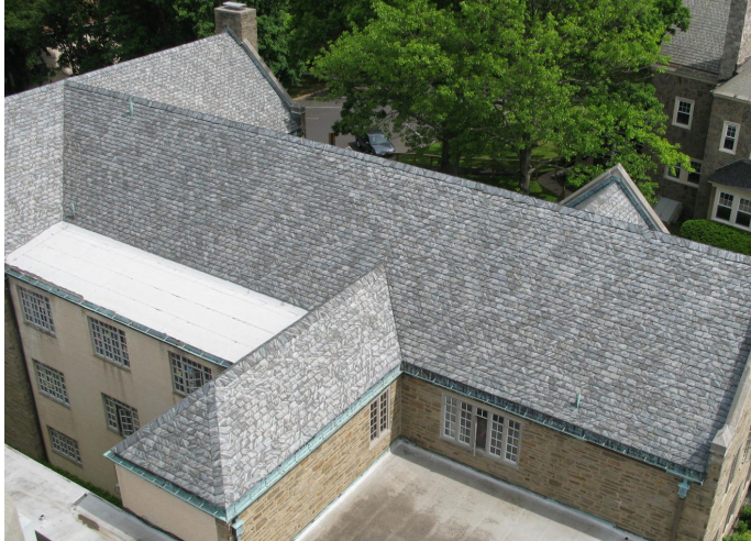
Figure 5: View of 80-year old Chapman slate on a roof in Glenside, Pennsylvania.
