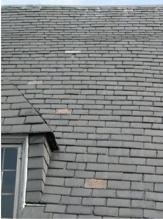
Figure 4: The five Pennsylvania Black slates used to repair this c.1924 Monson slate roof with varying exposures are not a good match. Three of the five replacement slates are nearing the end of their services lives (as evidenced by their surface delamination) and will need to be replaced yet again. (Interestingly, the varying exposures mentioned produced a wave effect when viewed from certain angles at grade.)
