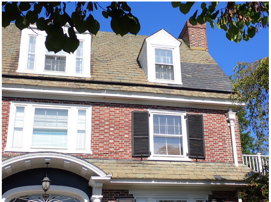
Figure 1: Mismatched Pennsylvania Black slate installed above the pole gutter on a New York/Vermont Semi-weathering Gray/Green slate roof.
